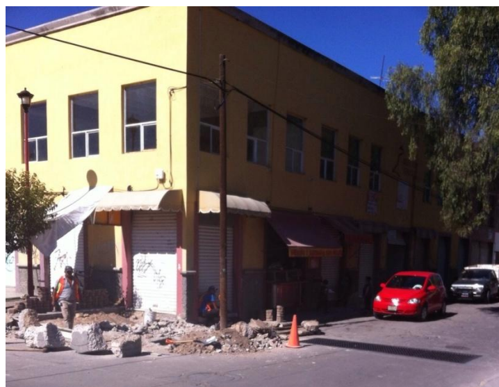
Figure 3: A taco local is located just next to the red car meanwhile there is a construction site next to it. There is no protection of any kind to avoid food contamination.
